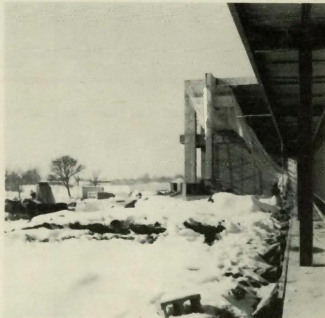
This partially completed Lexington ETV structure will be one of the finest in the United States. At the present time this building is only a skeleton, littered with concrete blocks and lumber—by Fall it will be complete and teeming with activity.
